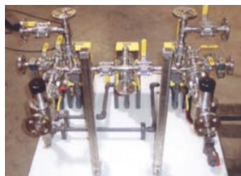
Chemical Feed Systems
